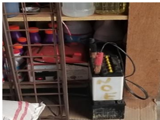
They utilize batteries to be obtain electricity. October 2018.
