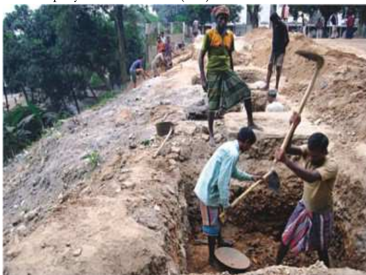
Figure 61 Digging for the construction of a multi-storied building ( www.thedailystar.net/news-detail-165276 , Published on November 2010 and Accessed on December 5, 2016)
