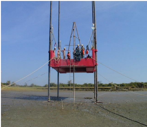
Photo - 5.3 Standing conditions on riverbed at Thilawa (No penetration into clay layer but not everywhere at Thilawa)
