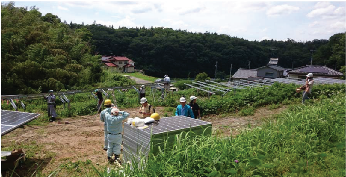
Figure A-2 Solar panel site in Kodani village
