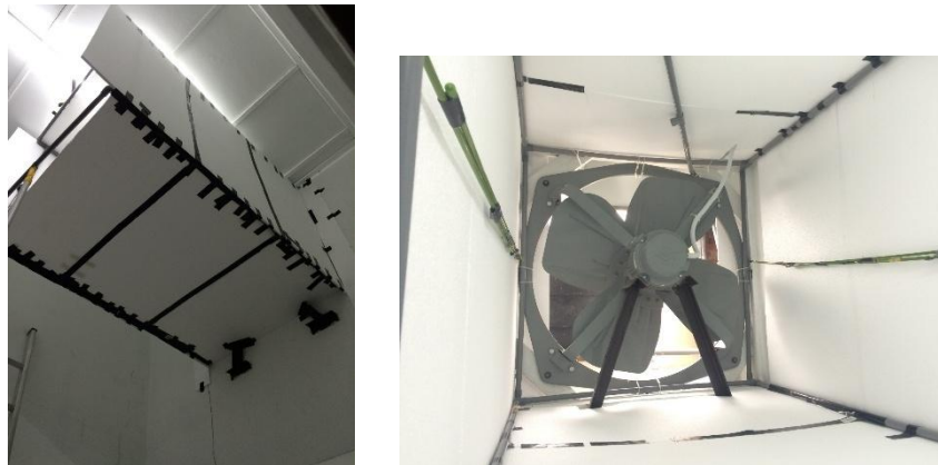
Figure B.1 Master bedroom fan and the whole house fan with the customized ducting system.
