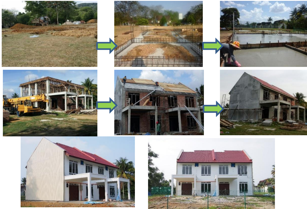
Figure 4.2. The construction process of the experimental house from site clearing until the completion phases.
