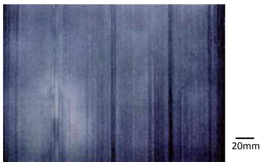
Fig. 3.5 Appearance of overlay welded panel in field test after 2 years
