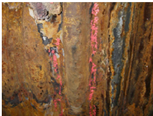
(a) Before de-scaling
