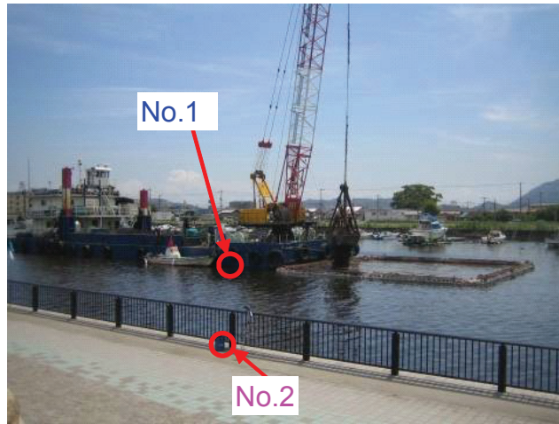
Fig. 4-2. pH monitoring sites during the construction. No. 1: Outside near the curtain to protect dispersion of silt (silt protector). No. 2: 20 m far from the curtain.
