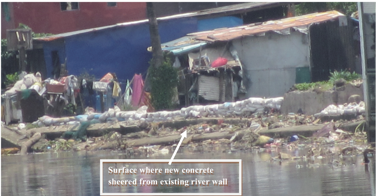
Figure 6. River wall collapse, sandbags provide temporary protection (Photo credit: Claire Pascua)
