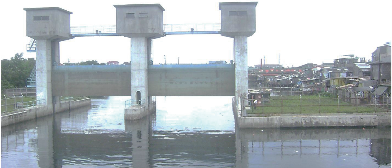
Figure 8. Raised C4 Floodgate (Photo credit: Arnel Tenorio)
