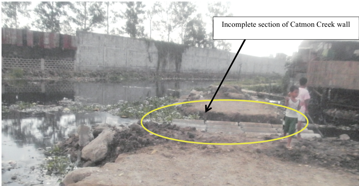
Figure 9. Incomplete Section of Catmon Creek Wall (Photo credit: Malabon City, 2012)
