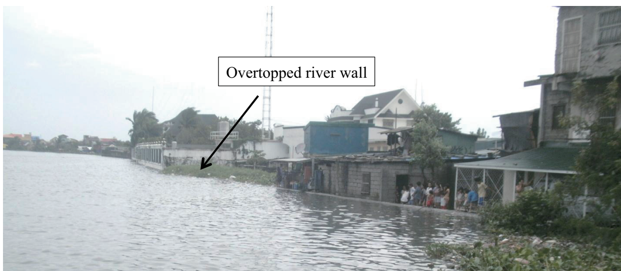
Figure 4. Tonsuya river wall immediately after Typhoon Gener (Photo credit: Malabon City, 2012)
