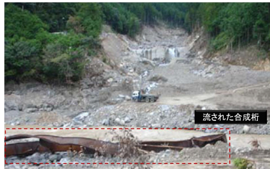
(b) A bridge broken by debris flow at 10.5.2011 (Photographer Dr. Kazuo Ishino in Taisei Kensetsu Ltd.)
