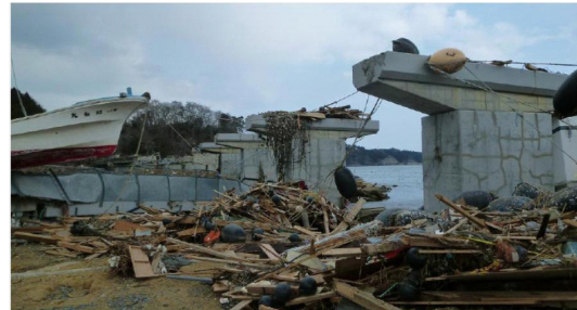
(a) A broken bridge by Tsunami at 3.11.2011
