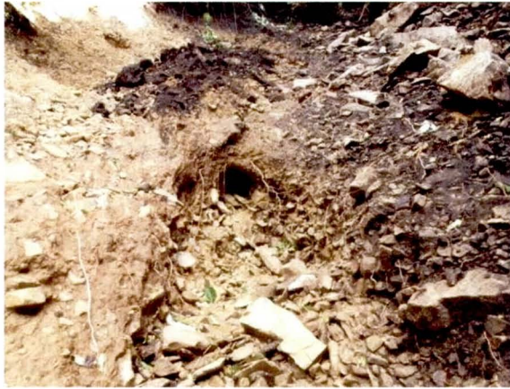
写真-5.2 崩壊源頭部のパイピング湧水 Photo 5.2 Piping-spring water at the head part of slope failure (図-5.22 中の①)
