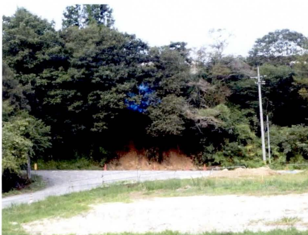
写真-4.11 道路沿いの小規模な崩壊 Photo 4.11 Small-scale slope failure along the road
