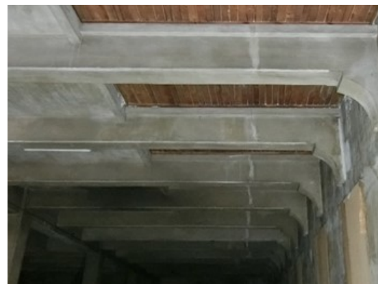
(d) Cracks in the same location on the second-floor beams
