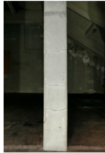
(b) Column with ring-shaped cracks (middle column on the third floor)
