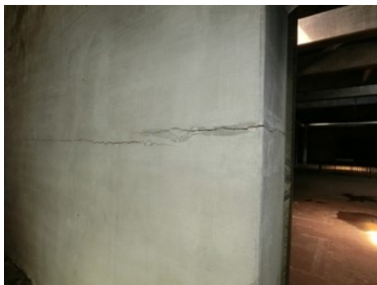
(c) Large horizontal cracks in the wall on the third floor
