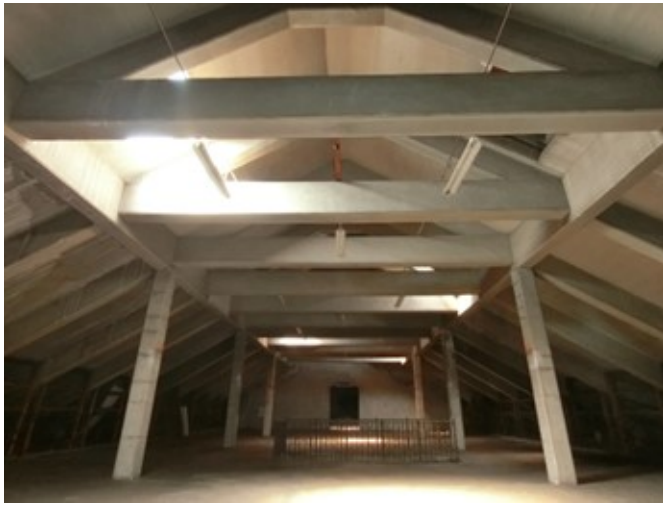
(a) Third floor with cracked columns
